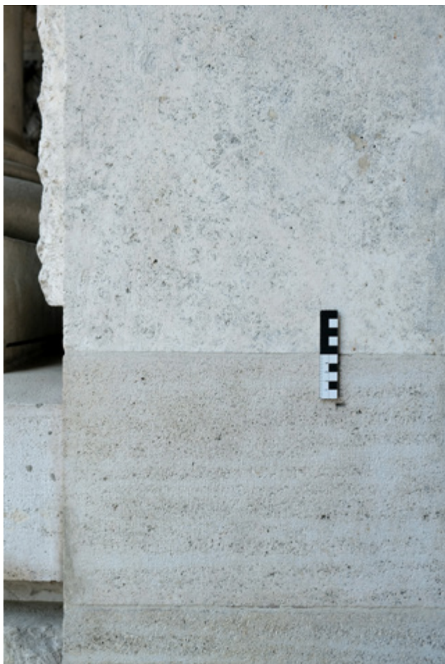
Fig. 8. Detail of door soffit–Wöllersdorfer at the lower part and Pula limestone at the upper, 2022
